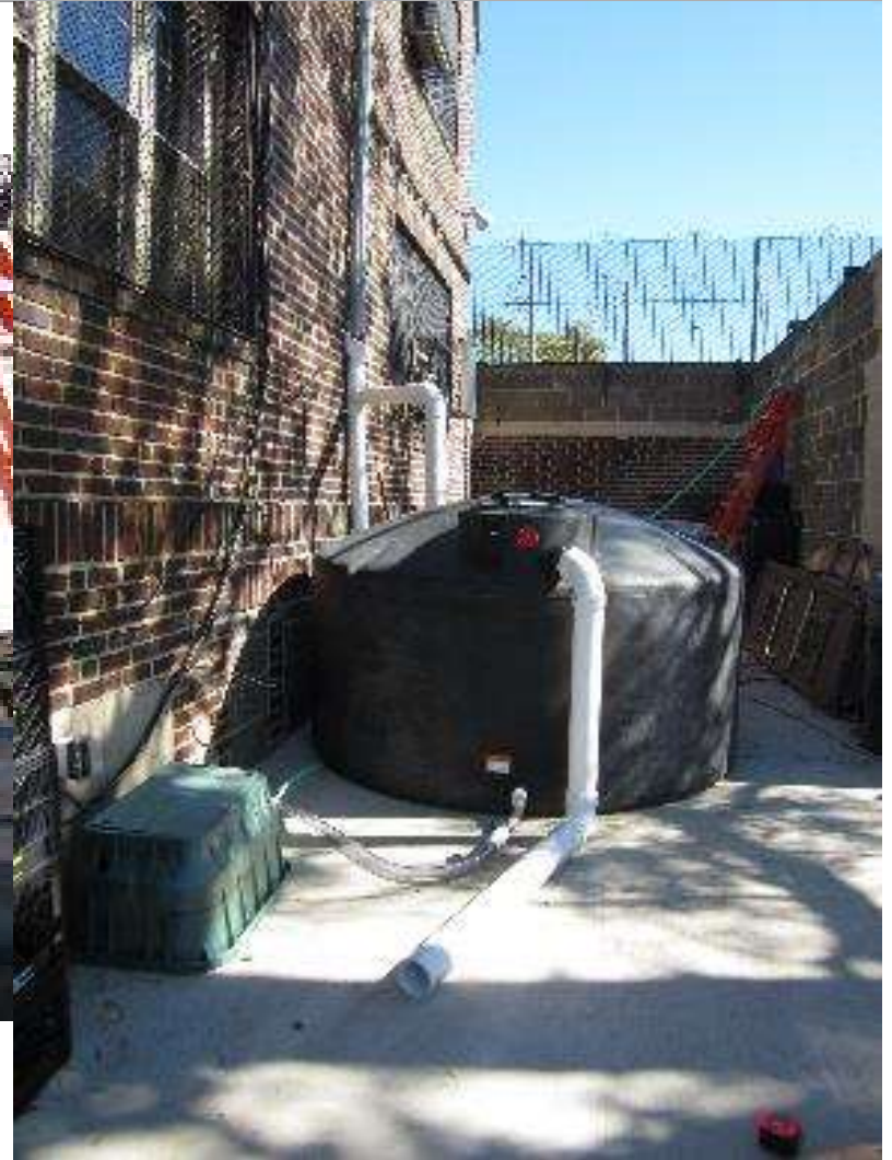
Cistern at the Neighborhood Center in Camden, NJ Harvesting System
