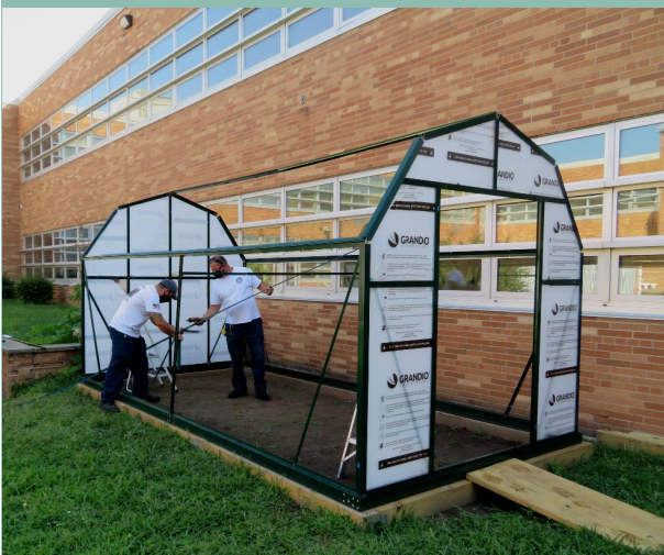
Marco Canova, Equipment Operator II, and Scott Scardilli, Equipment Operator I, from the River Restoration Department, working on the Harrison Middle School Greenhouse.
