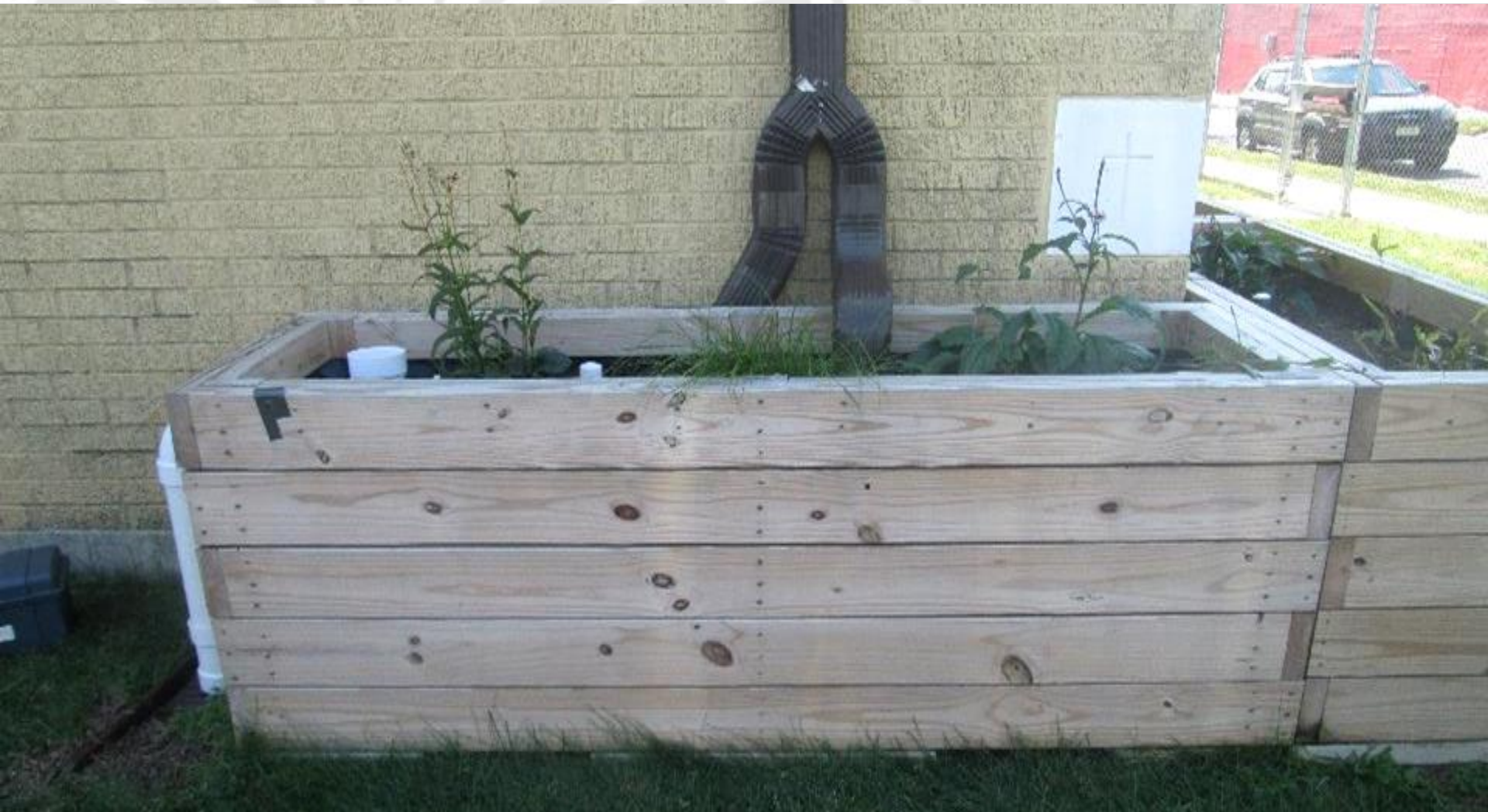
Downspout Planter Boxes at Acelero Learning Center in Camden, NJ Harvesting System
