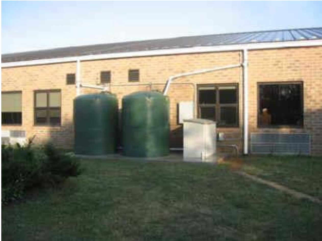
Samuel Mickle School Rainwater Harvesting System
