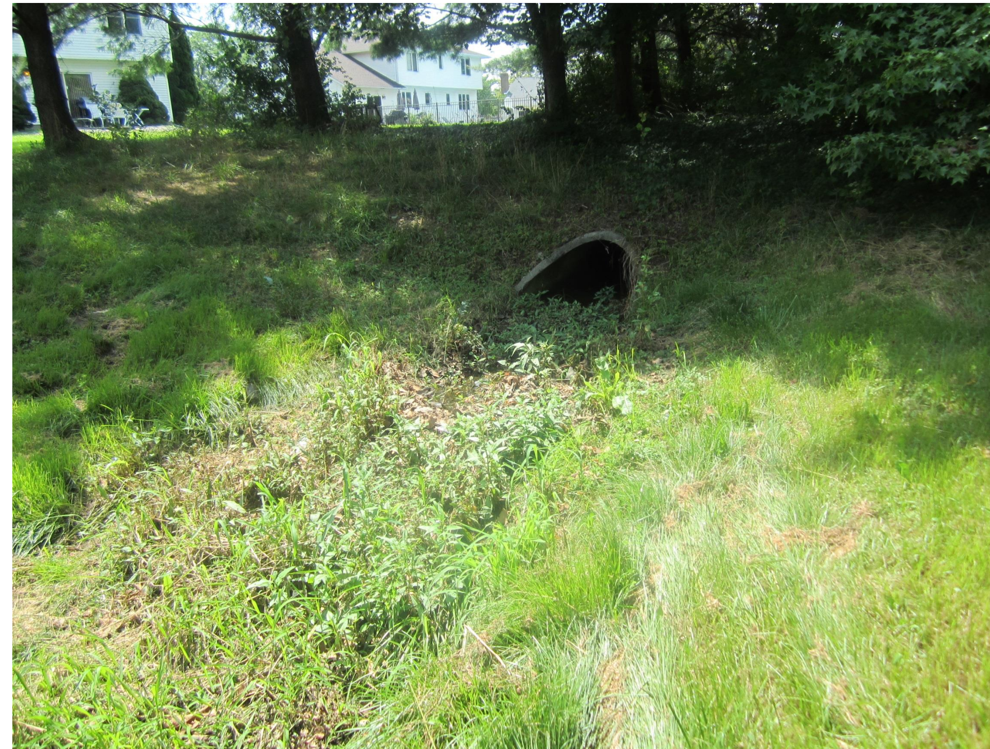
Excessive sediment in front of inlet
