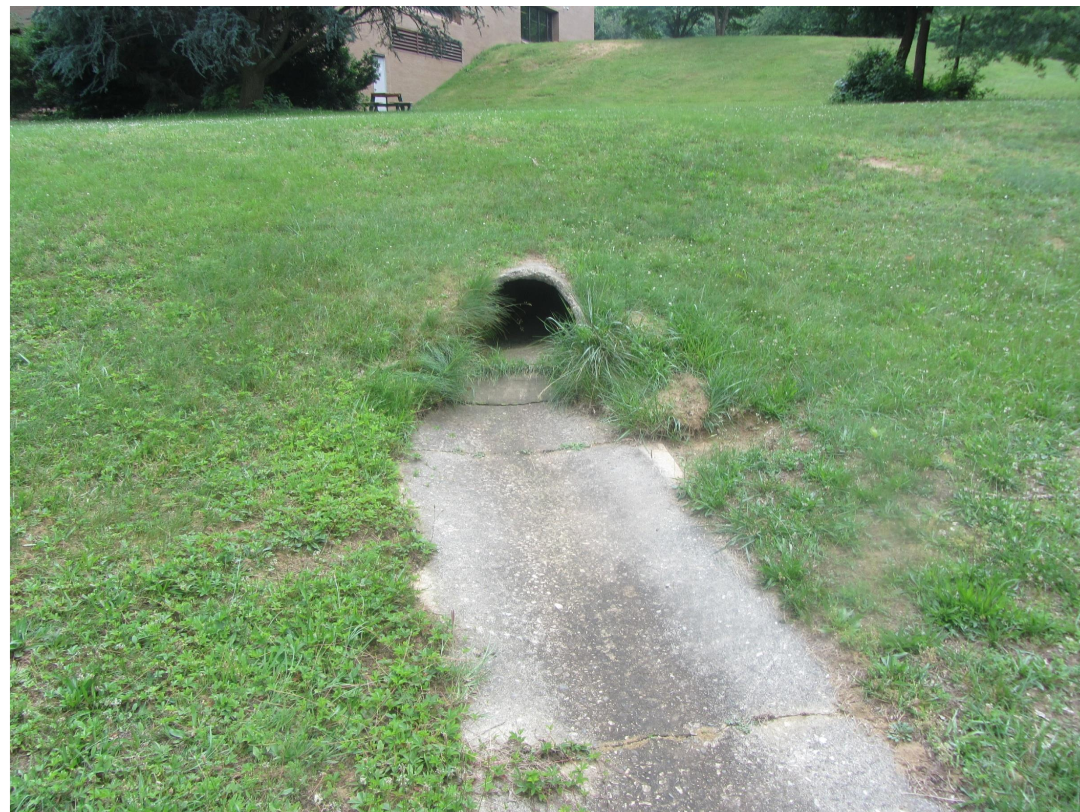
Concrete deterioration on northern inlet
