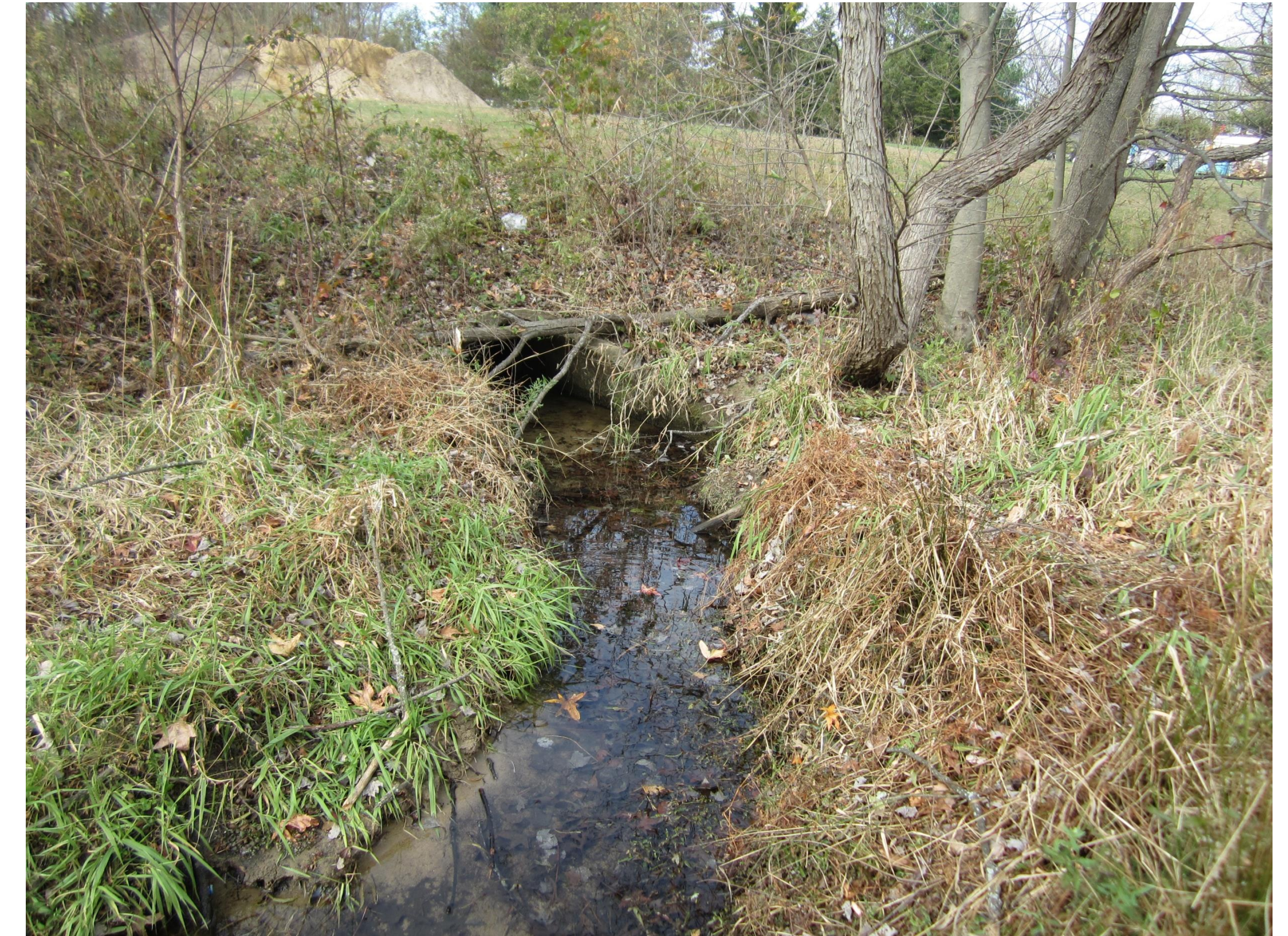
Inlet and erosion
