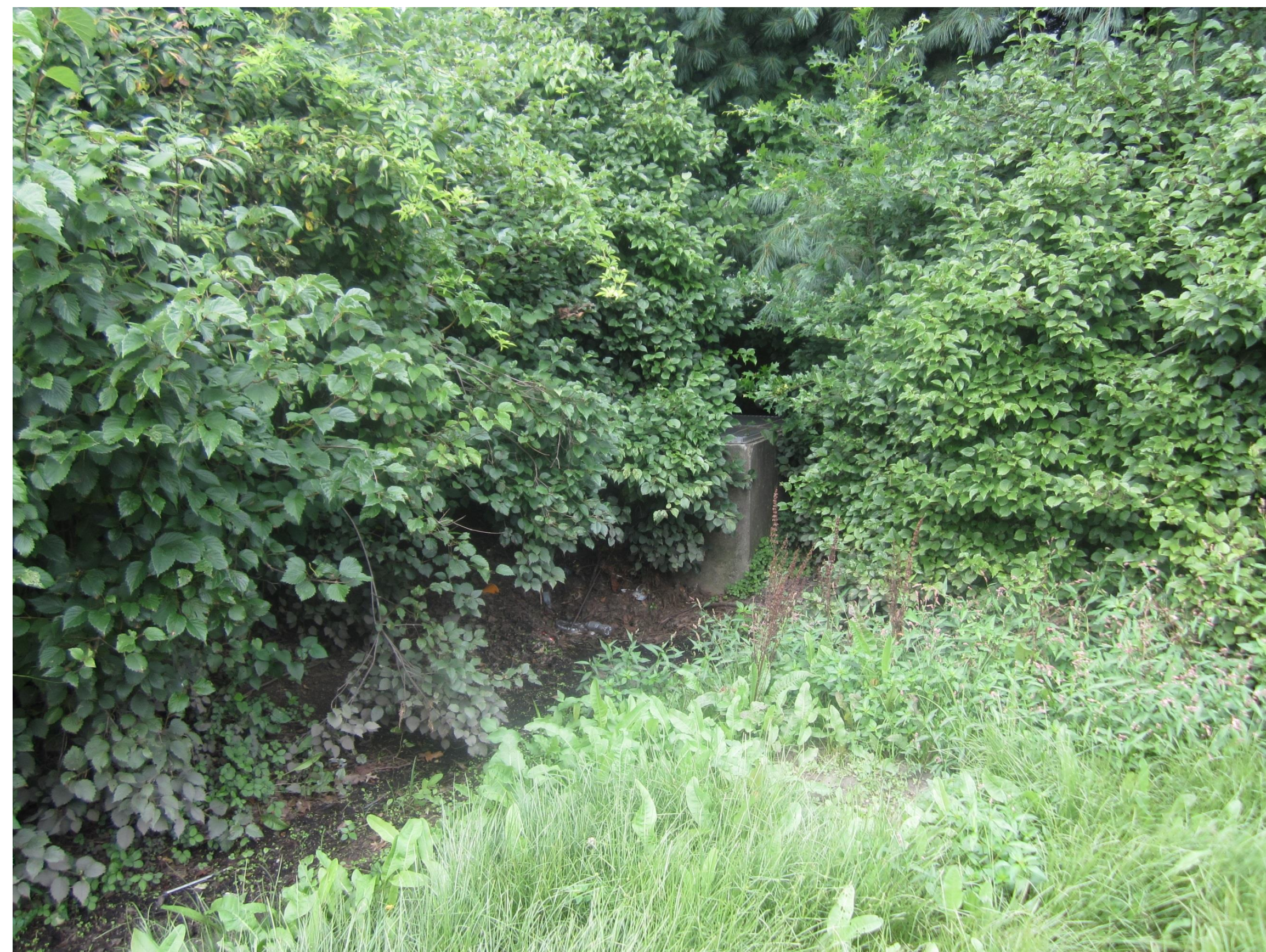
Overgrown outlet structure
