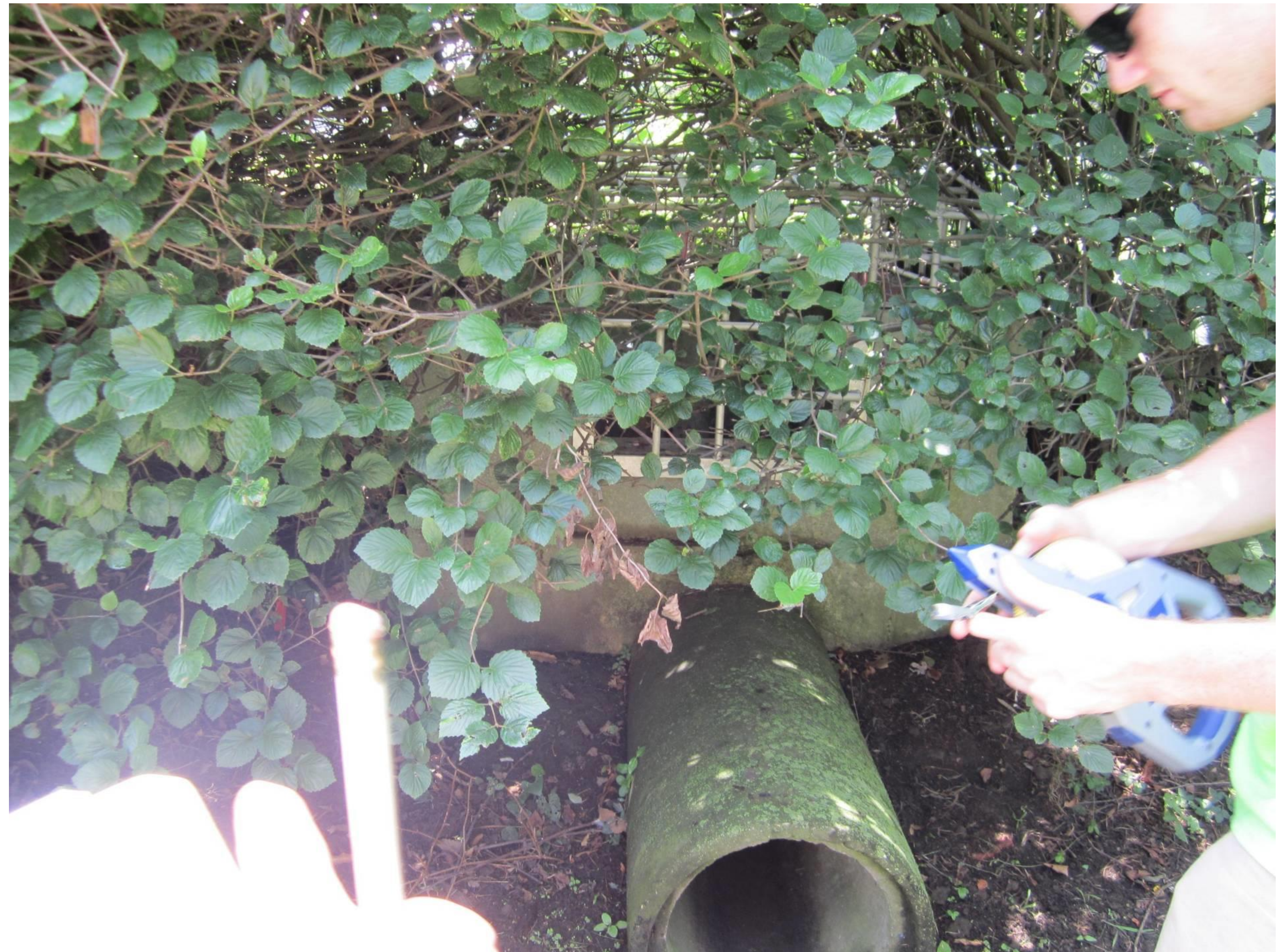
Woody vegetation growth around outlet
