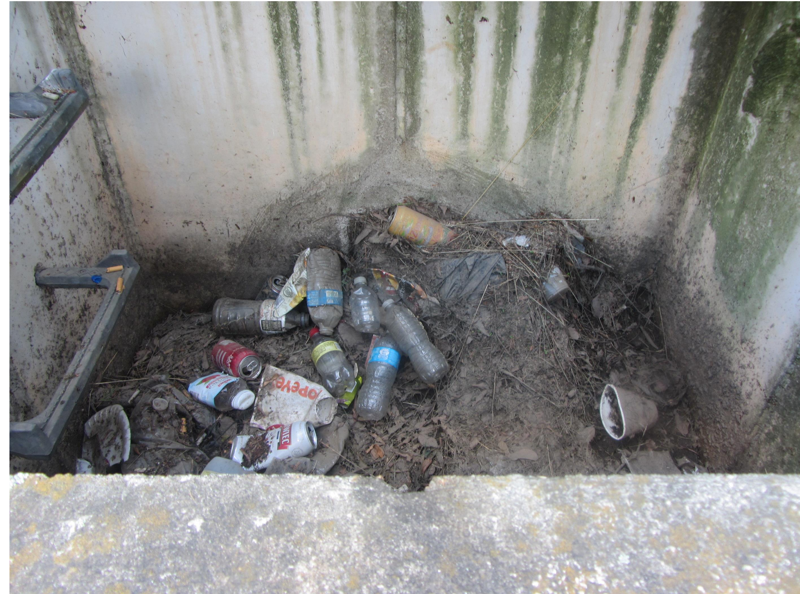
Litter and debris accumulated inside outlet
