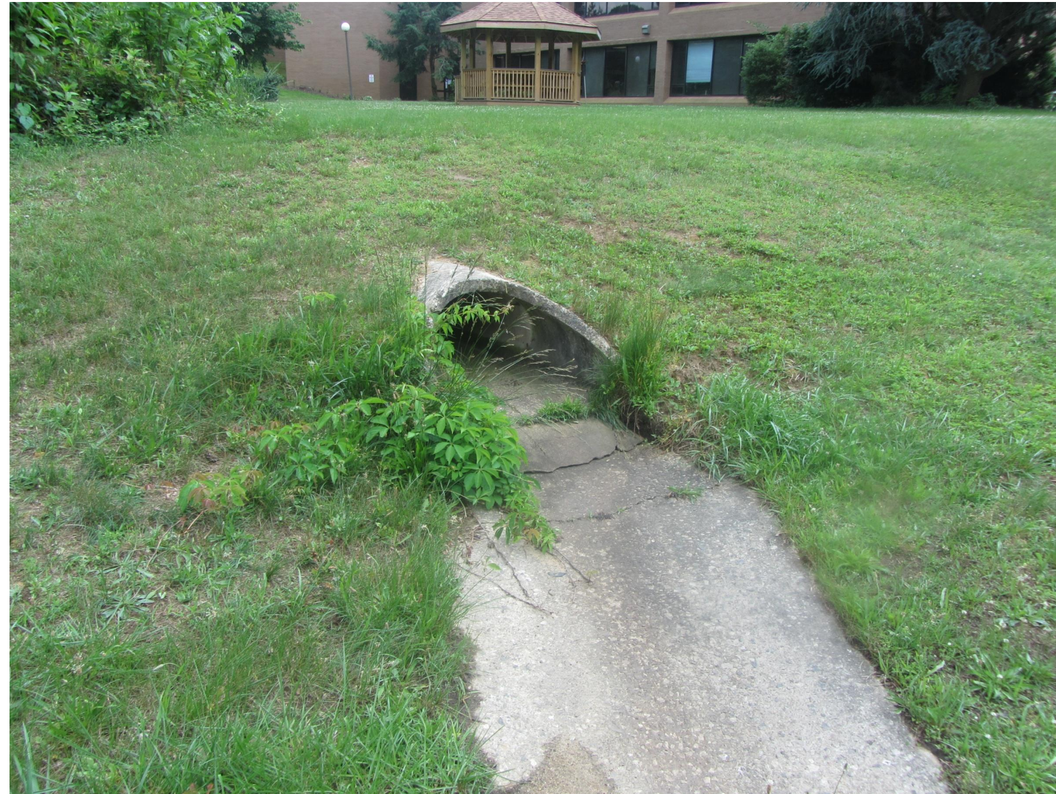
Concrete deterioration on southern inlet
