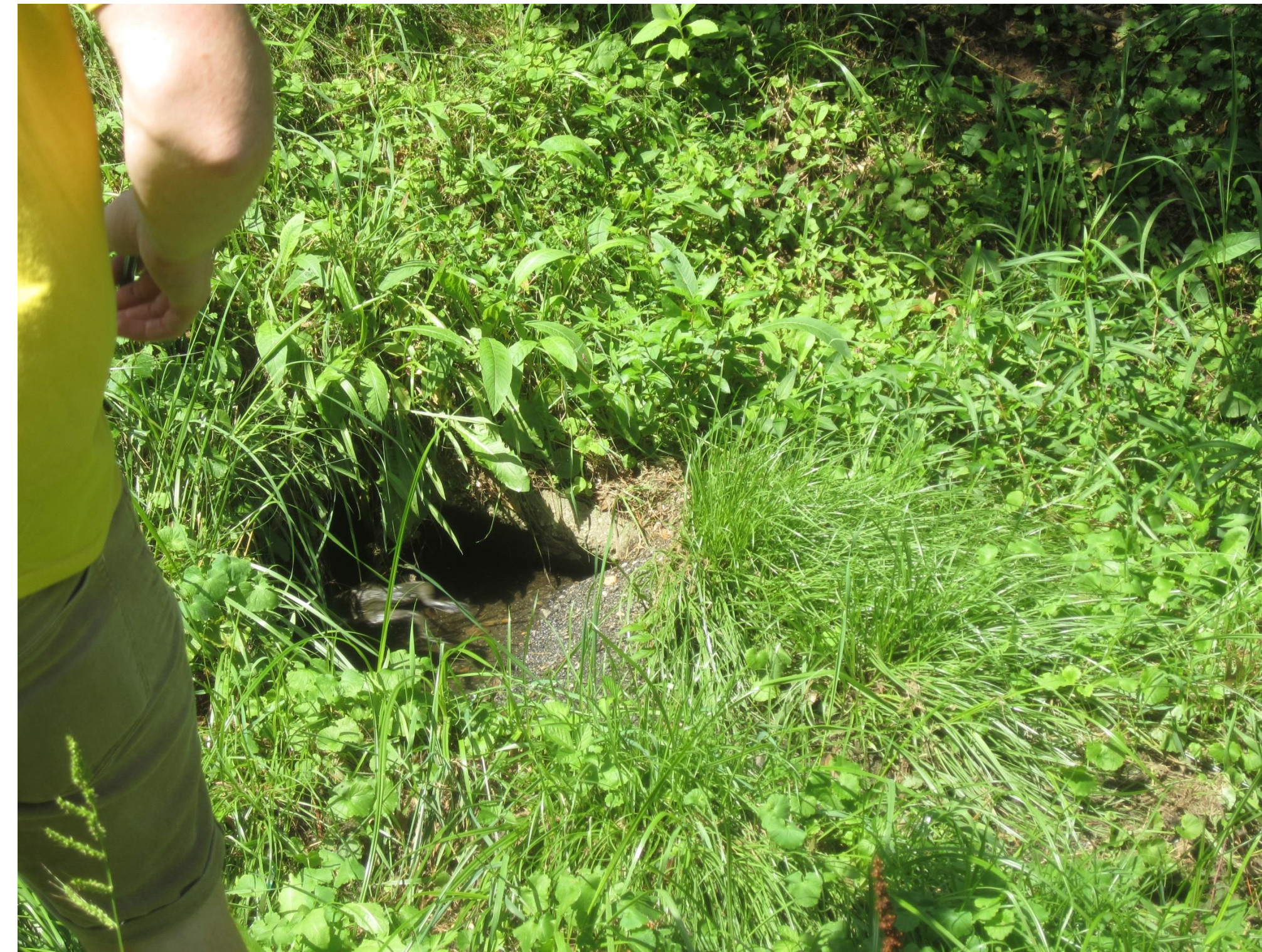
Southern inlet structure filled with sediment
