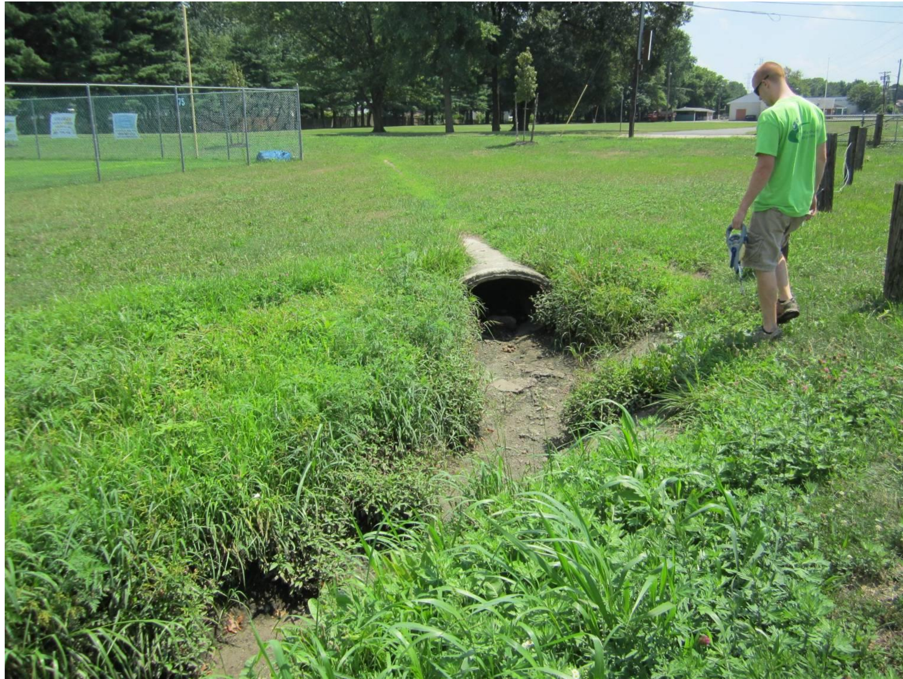
Inlet with sediment accumulation
