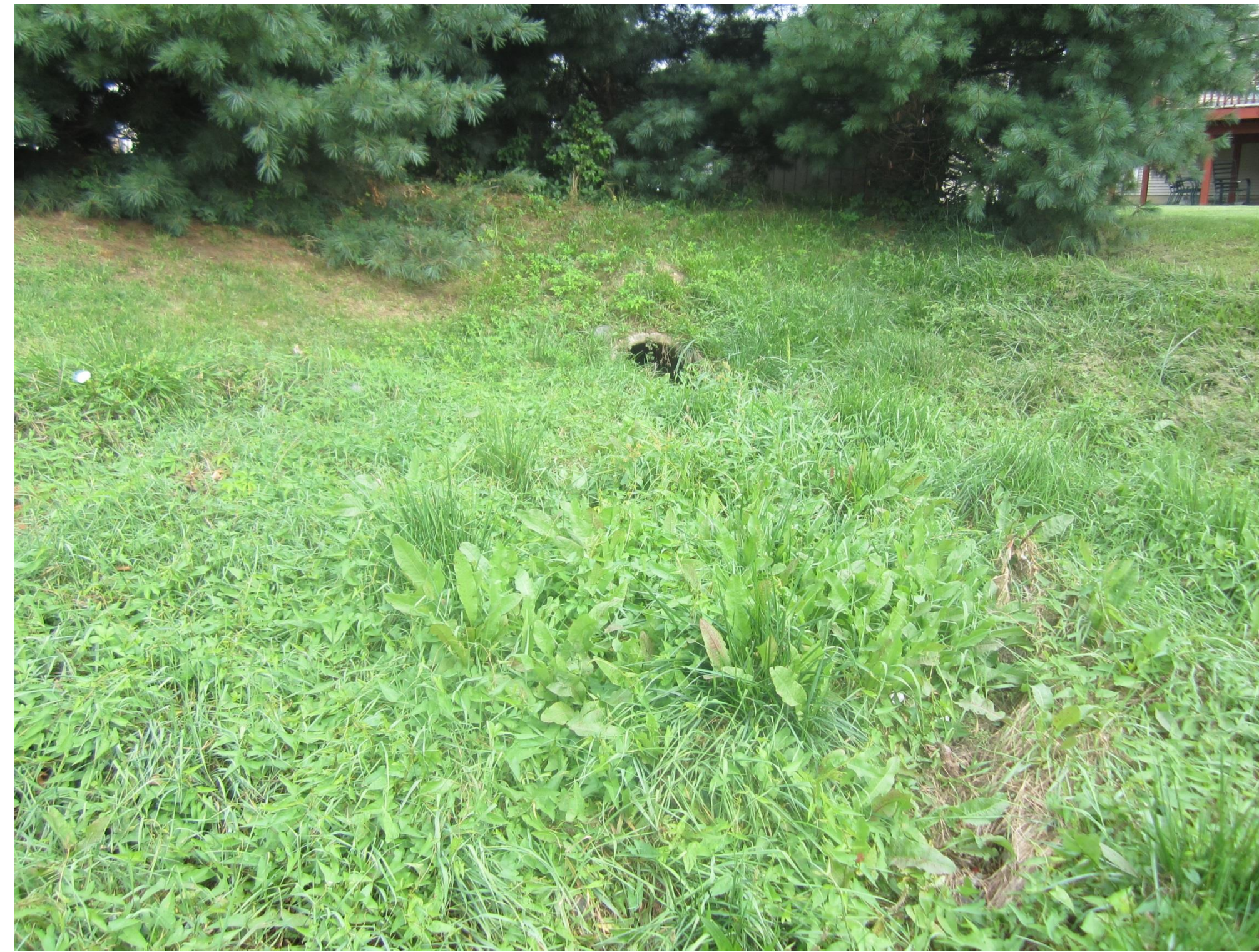
Inlet structure and overgrown rip-rap apron
