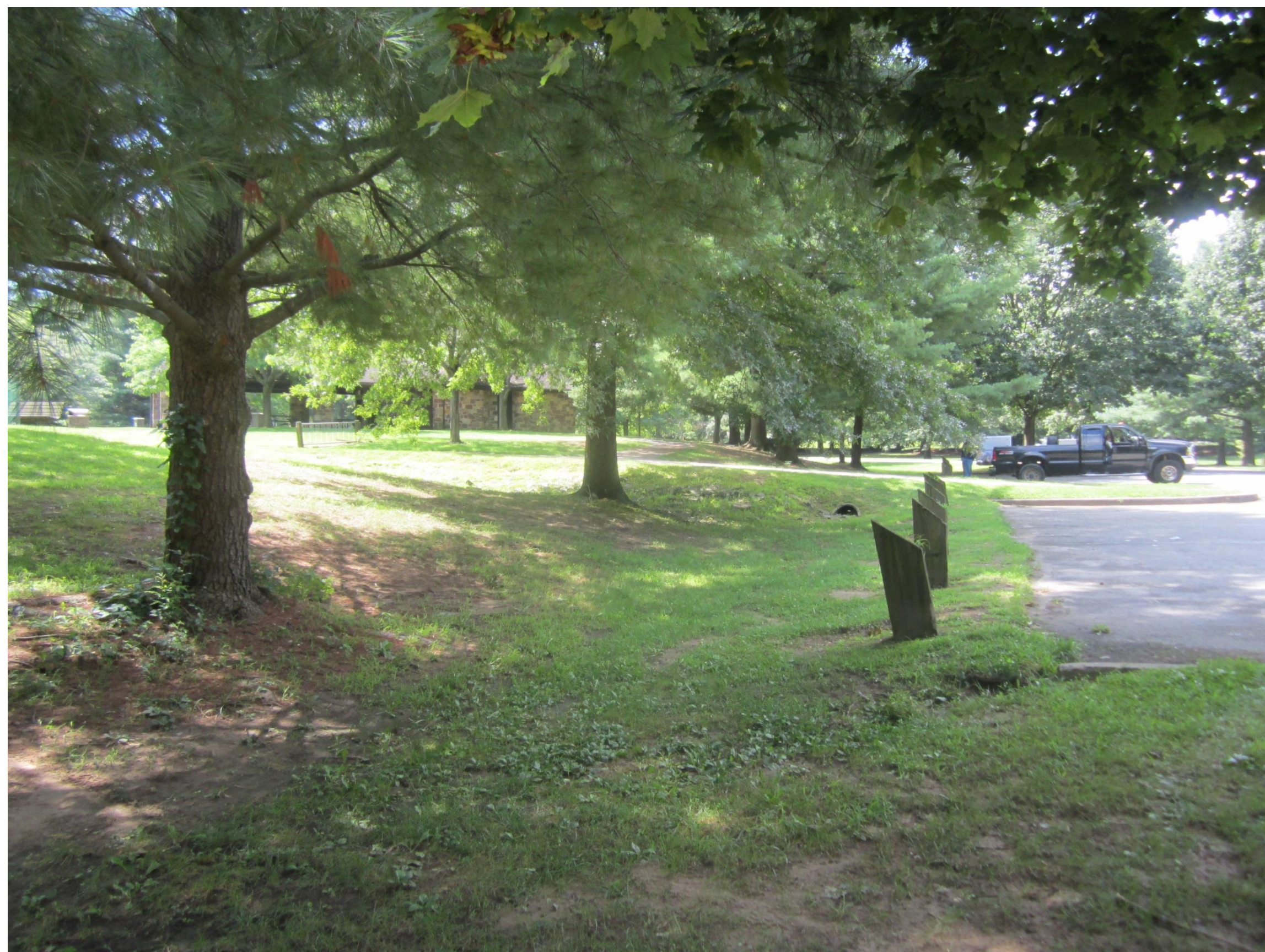
Swale that conveys two inlets to basin
