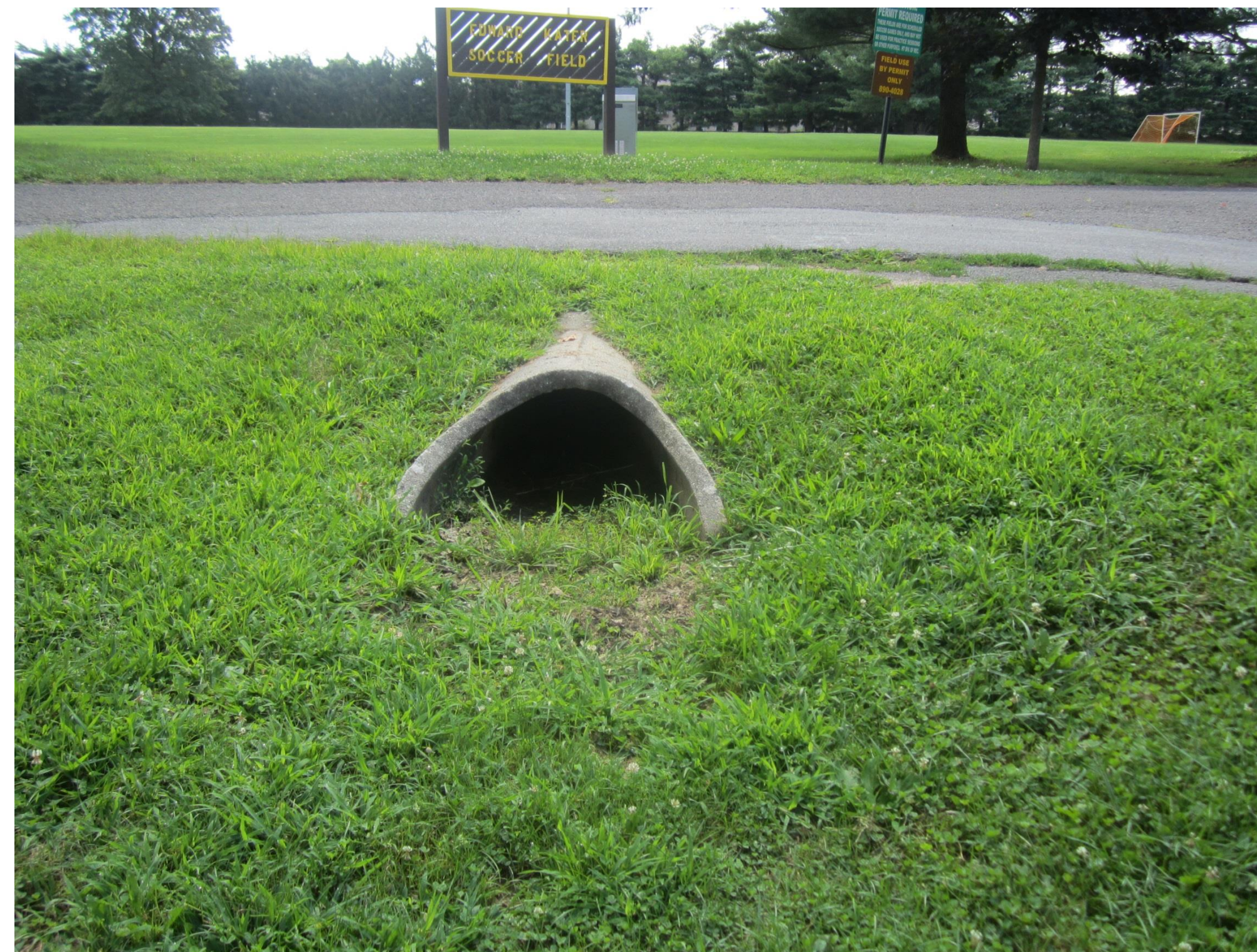
Basin #159 inlet structure
