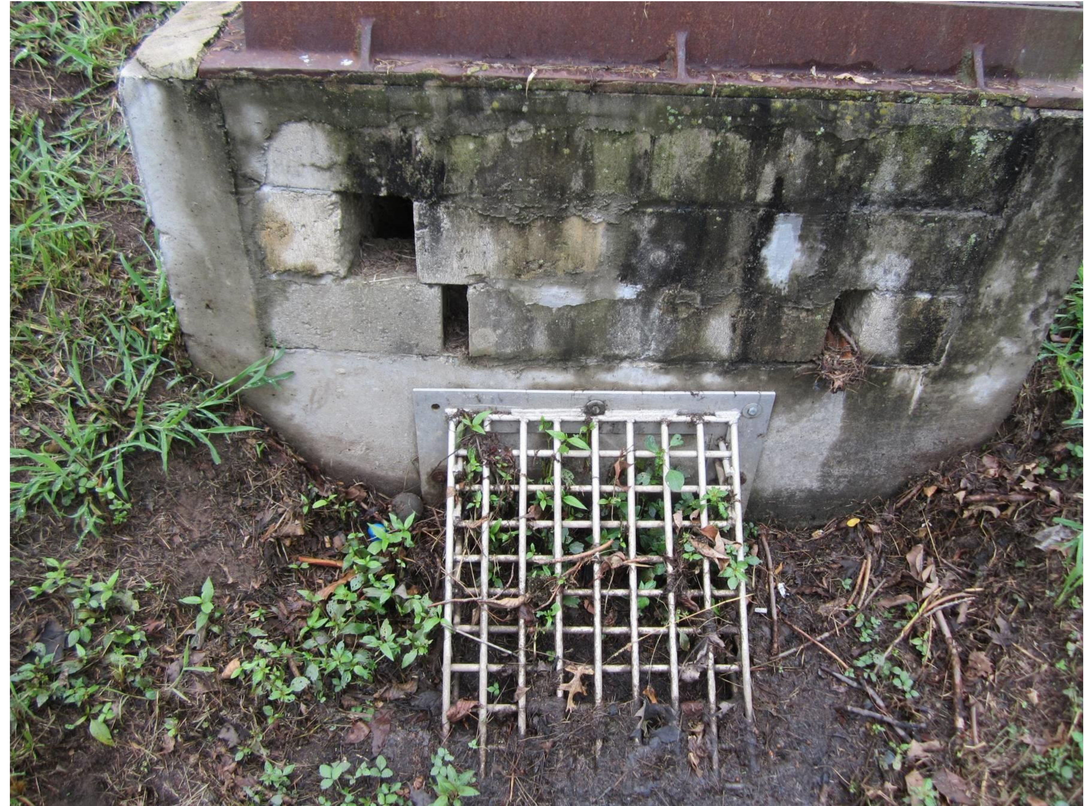
Clogged trash rack at outlet
