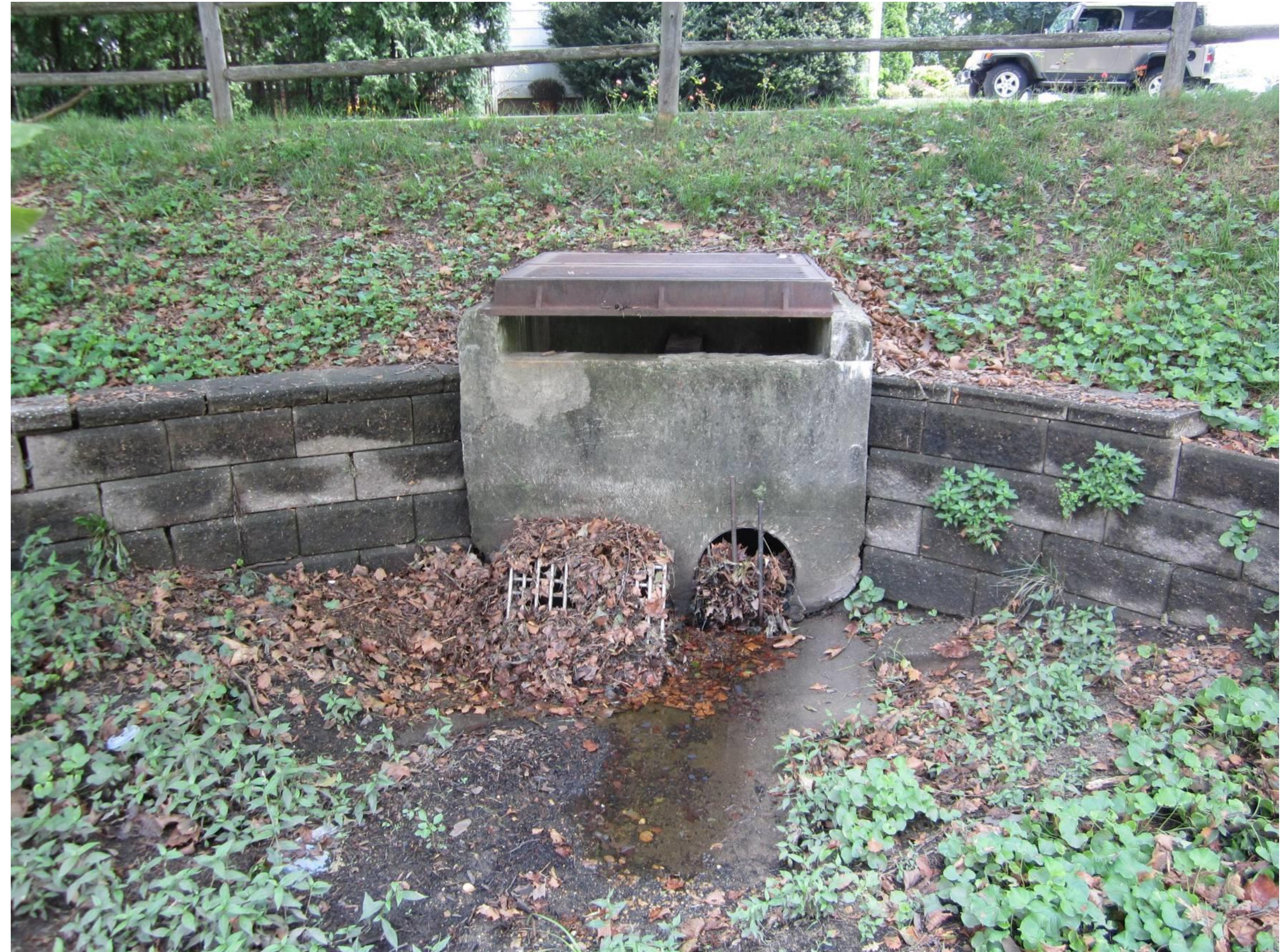
Clogged outlet structure
