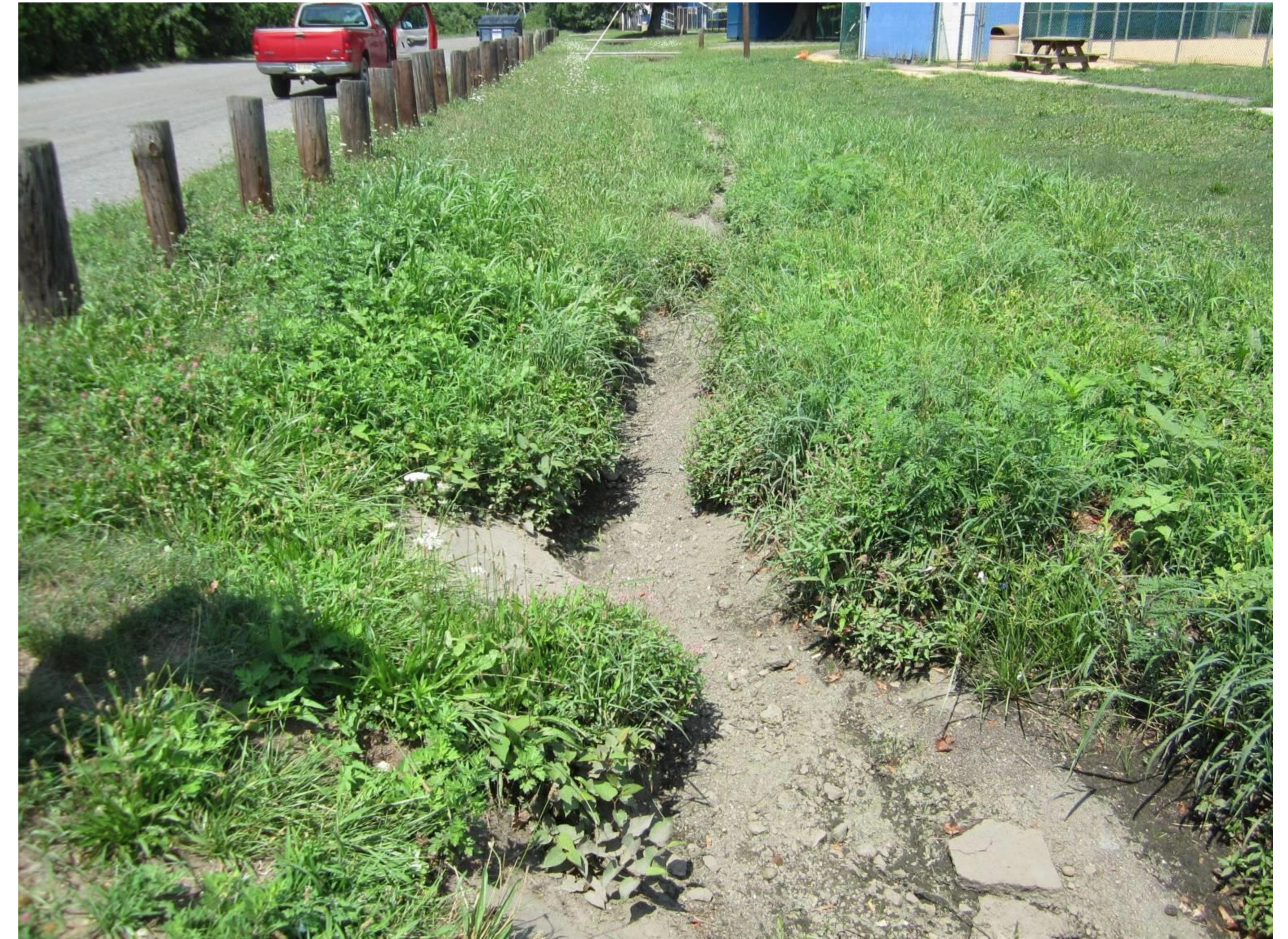
Basin bottom with erosion
