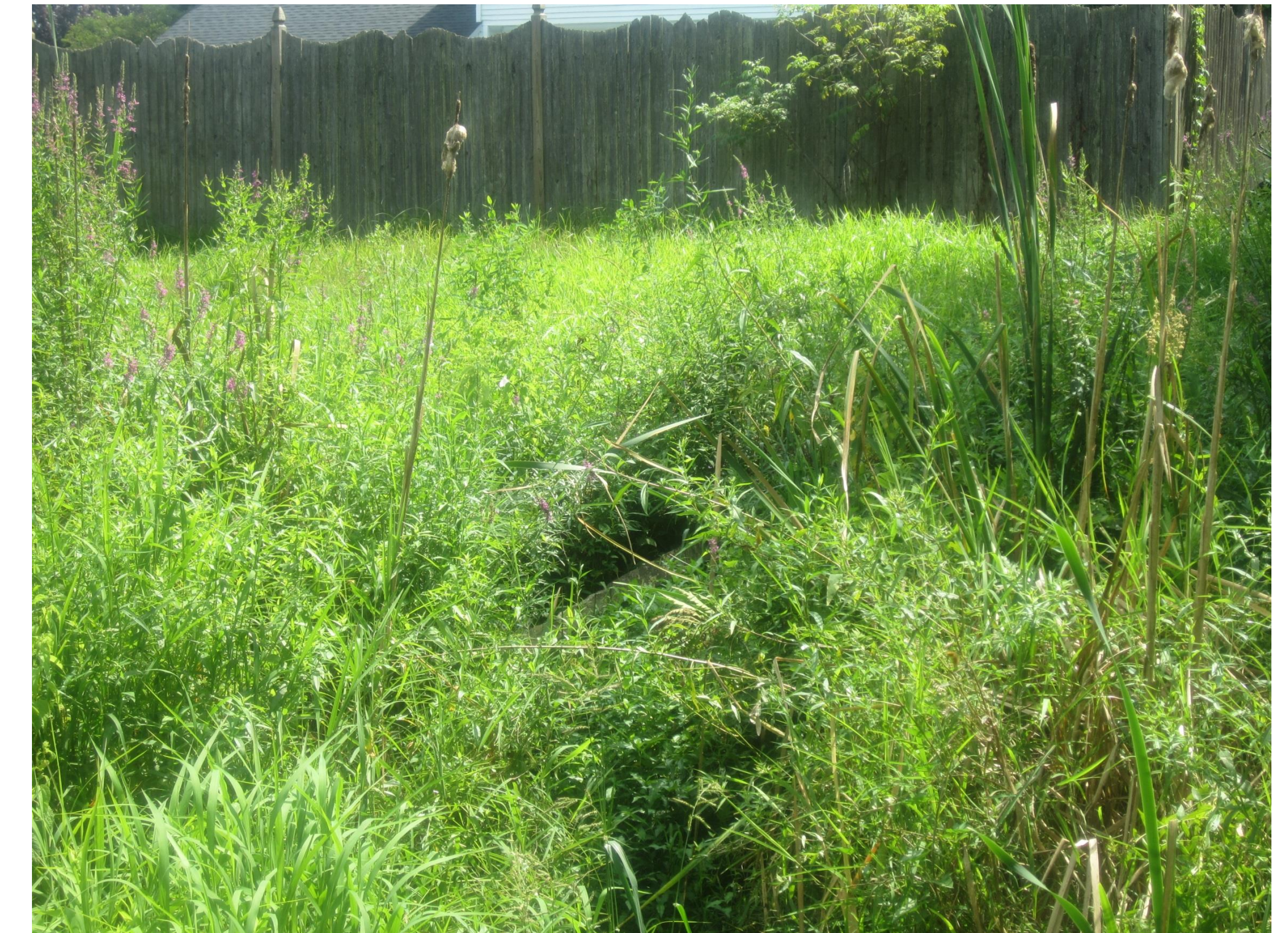
Overgrown western inlet
