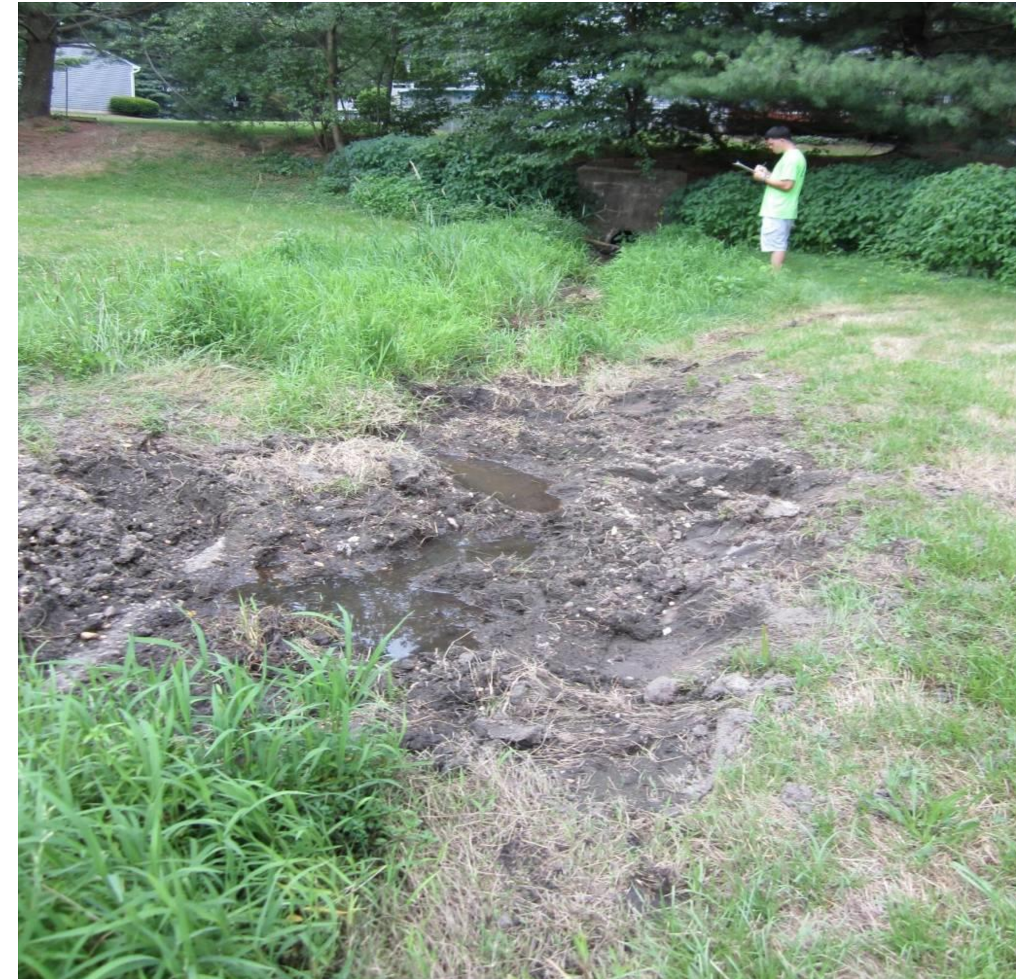
Clogged low flow and outlet.
