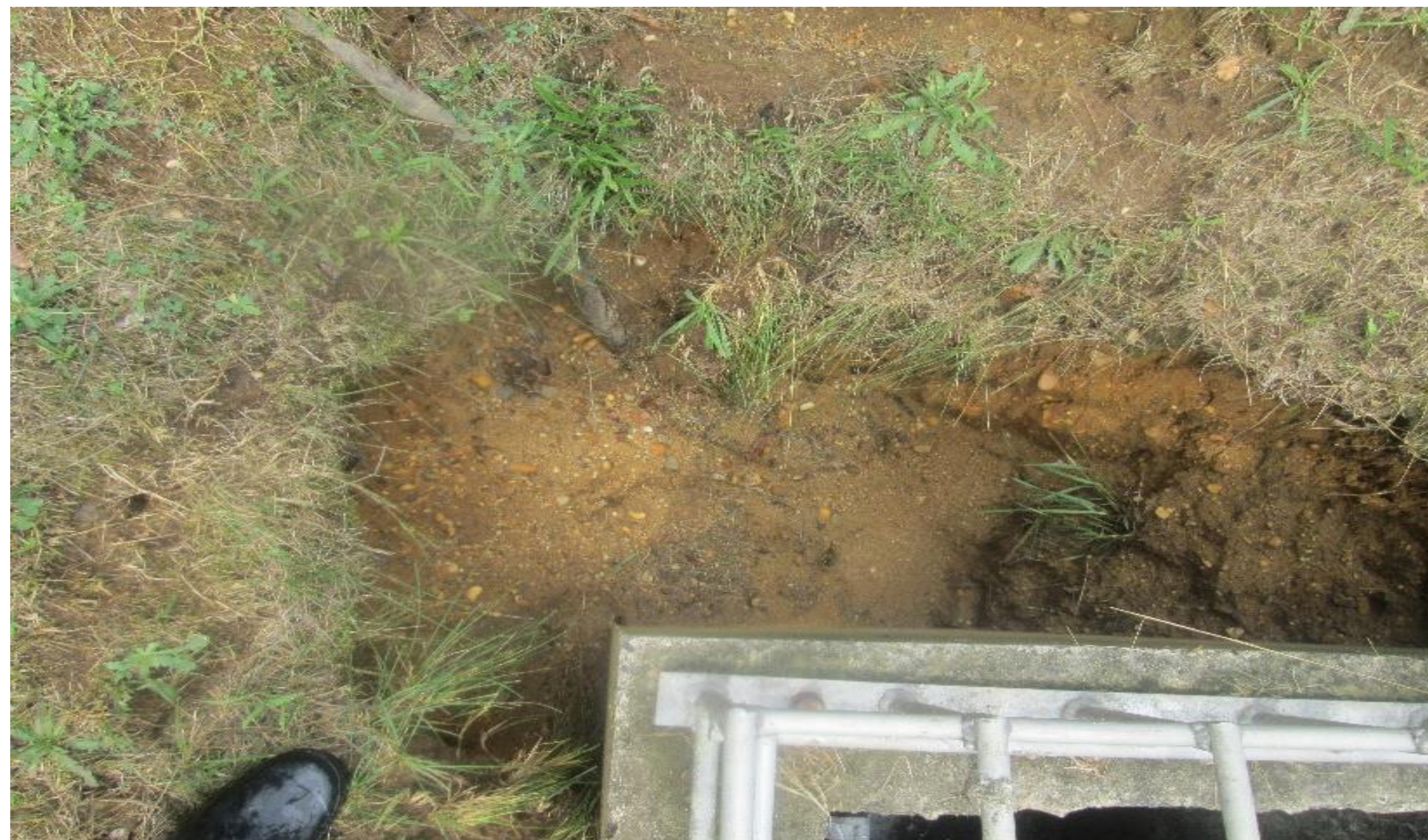
Erosion near outlet structure
