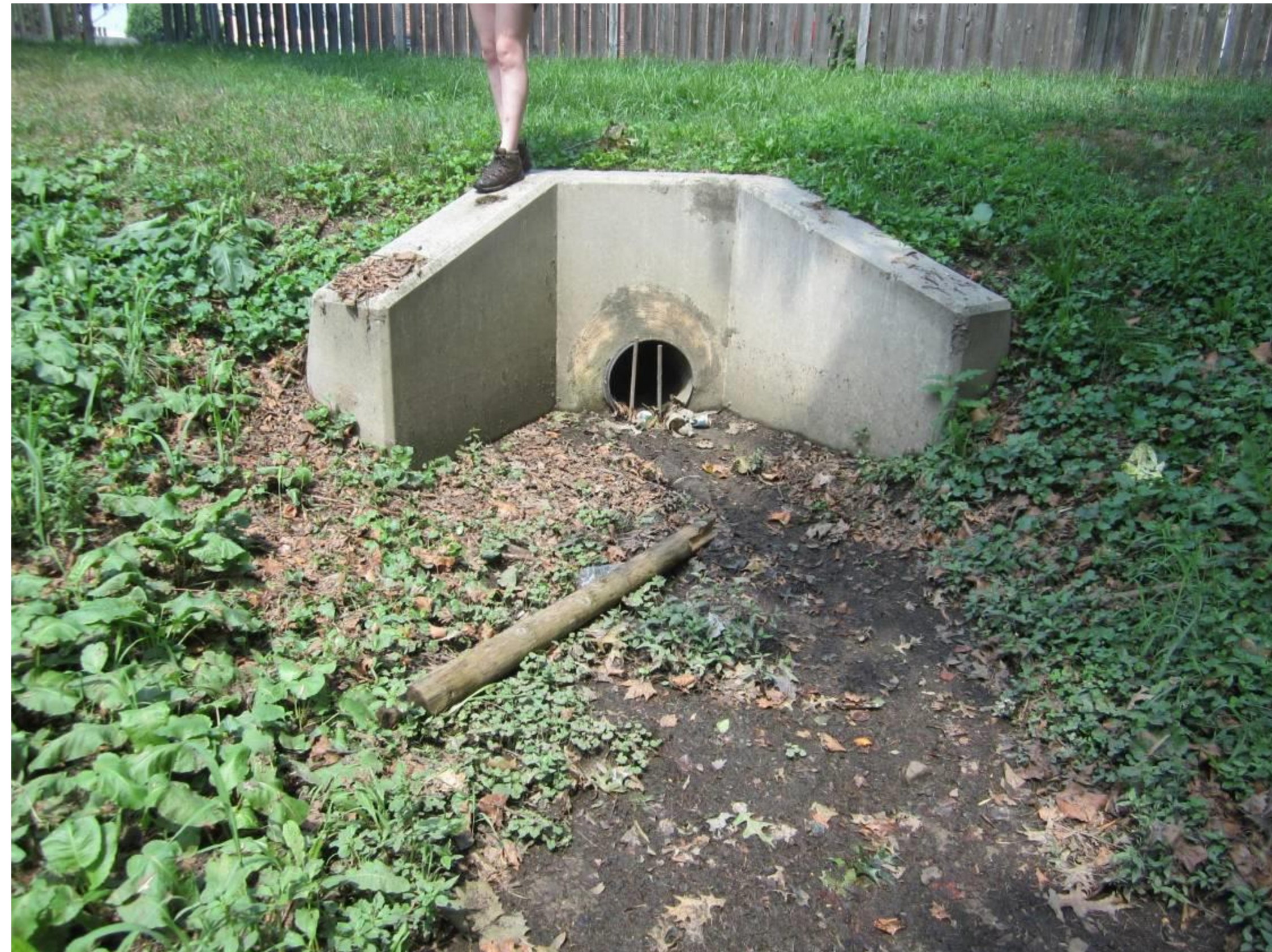
Inlet clogged with sediment
