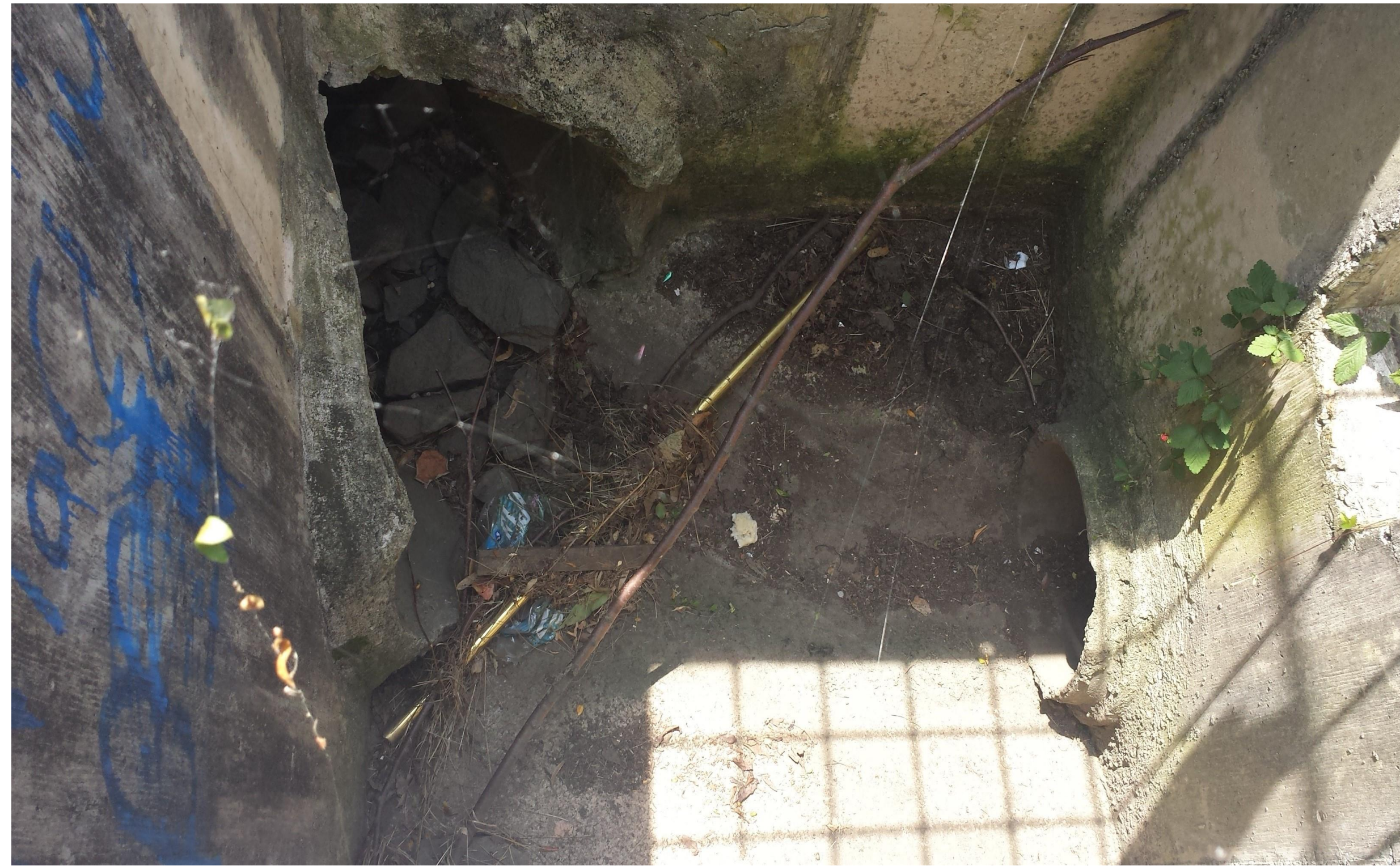
Inside of outlet
