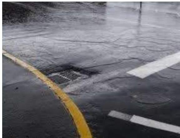
Figure 1: Stormwater draining from a parking lot
