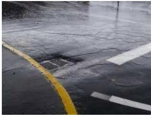
Figure 1: Stormwater draining from a parking lot
