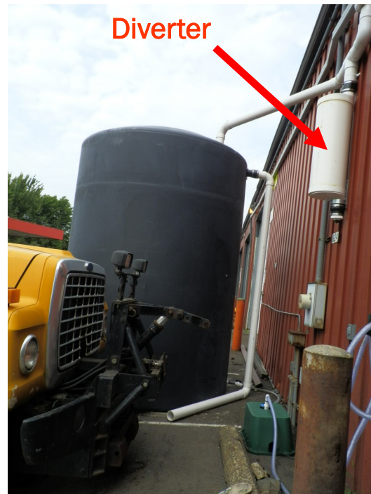
Cistern at Parsippany Troy-Hills DPW facility with diverter Photo credit Pat Rector
