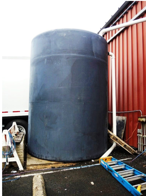
5,000 gallon cistern installed at the Parsippany-Troy Hills DPW yard capturing roof runoff from the main building on site. Photo by Ed English
