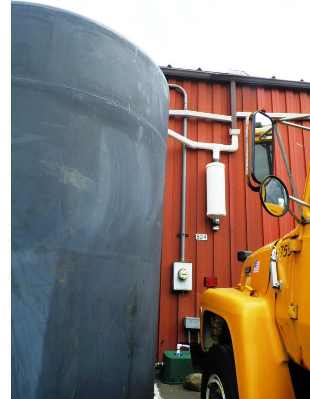
Close up view of cistern and diverter. Photo credit Pat Rector
