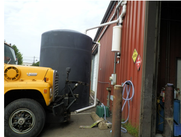
The cistern at the Parsippany-Troy Hills DPW. This water is used for truck washing and to fill street sweepers. Photo credit Pat Rector
