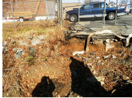
This area at the mouth of the vegetated swale of the Parsippany Troy-Hills DPW was excavated by the DPW staff to install sedimentation chambers. Photo credit Pat Rector
