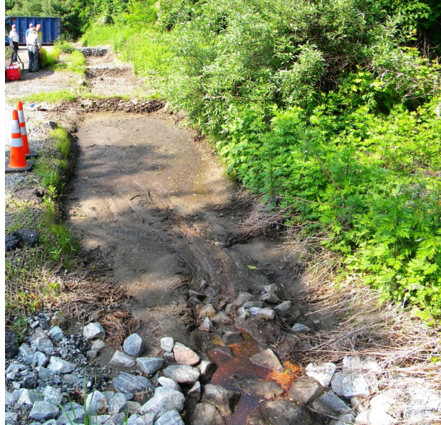
Vegetated swale (1,200 linear feet) with the first cell filled with sediment. Photo credit Pat Rector
