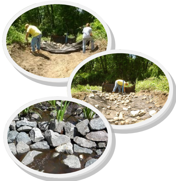
The rip-rap apron at the outlet provides for final settling and velocity reduction prior to entering the Troy Brook.
