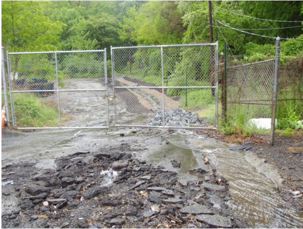
A 66,300 square foot parking lot drains to one area bringing dirt from truck washing and other normal operating dirt along with some residual hydrocarbons from fueling station.
