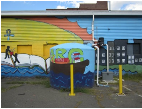
A cistern to store rain water was installed at Paterson School #5 for its community garden
