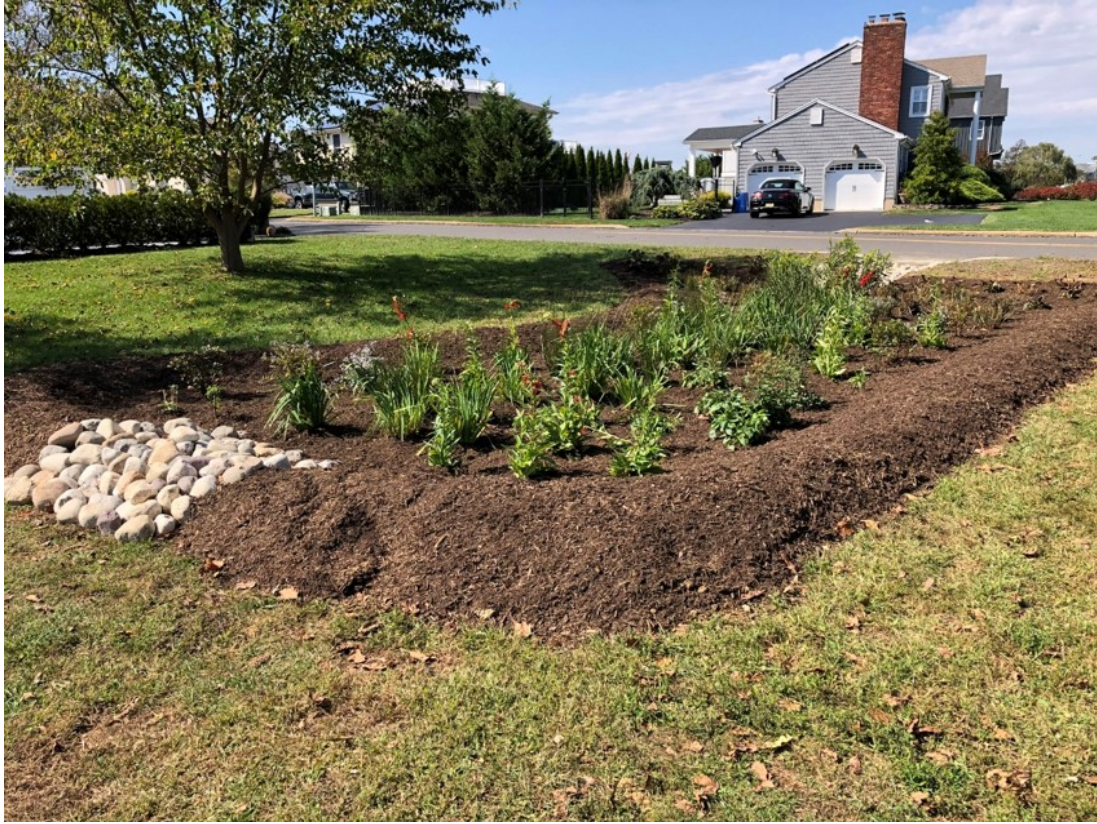
Monmouth Beach rain garden following planting, October 2020
