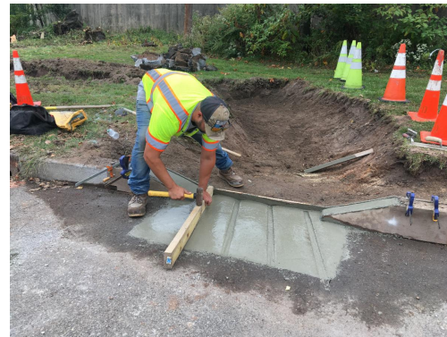
Curb-cut for Fulton Street rain garden #4, Woodbridge, NJ
