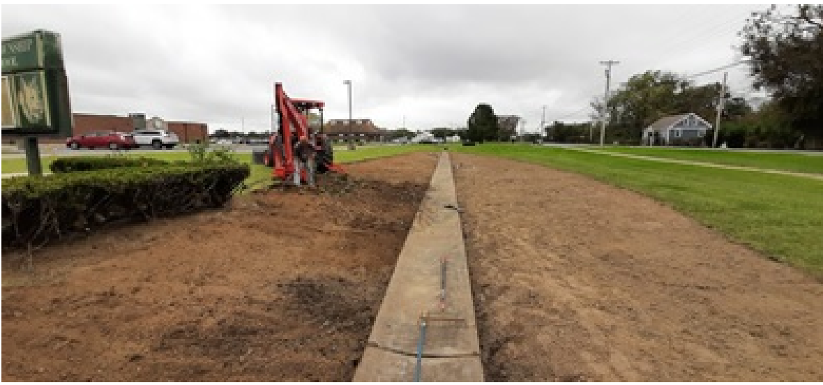
Phase 2: Removal of sod to retrofit the basin at Pittsgrove Township Middle School, October 2021
