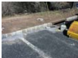
Sources of nonpoint source pollution such as road salt buildup near this stormwater grate can be identified in a watershed assessment.
